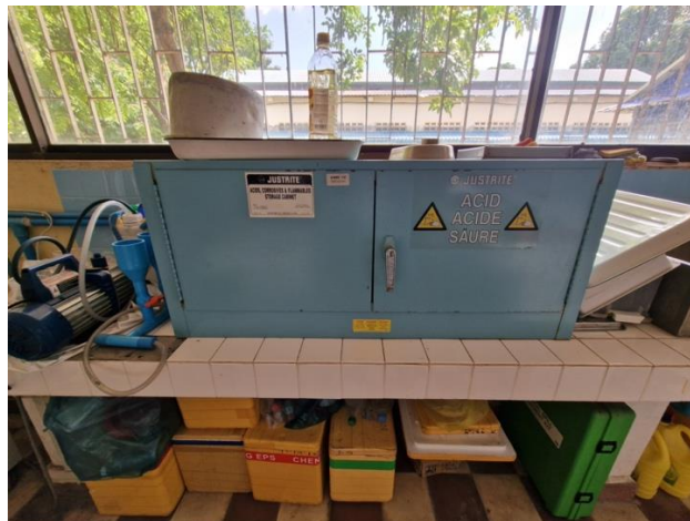
Figure 7: Metallic closet for acid, corrosive and flammable products at RUA laboratory.
